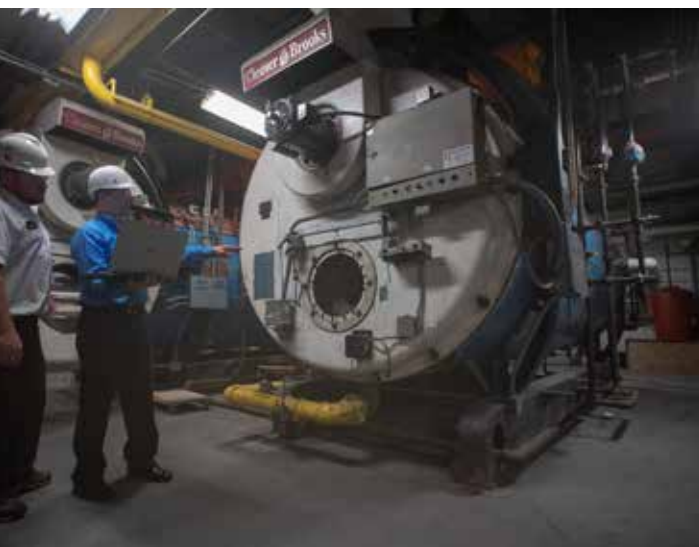
Building Chief Engineer Joe Tracy and IBS Sales Engineer Joe Crosetto evaluate the existing mechanical equipment
